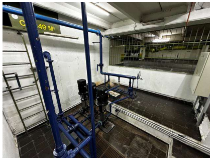
SALA BOMBAS AP
